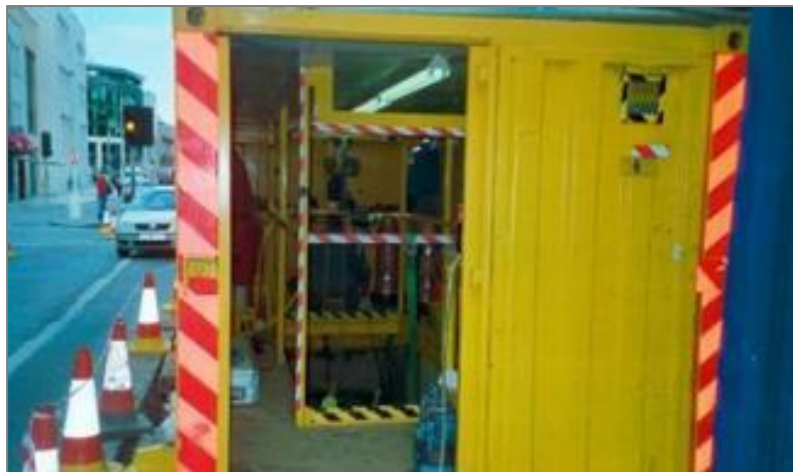
Figure 11 - HV cable jointing container
